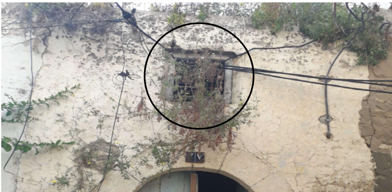
Distribution / armoire non conforme
